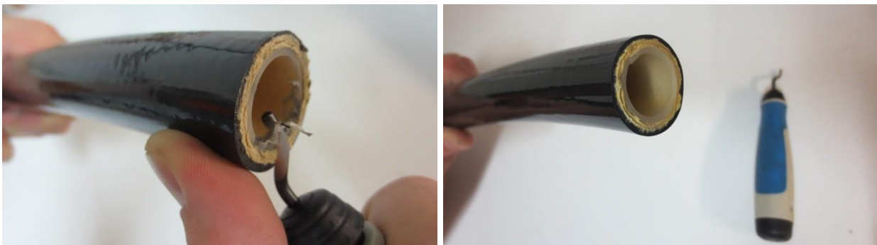
Use a proper tool to remove burrs and/or residual from the cut surface.
